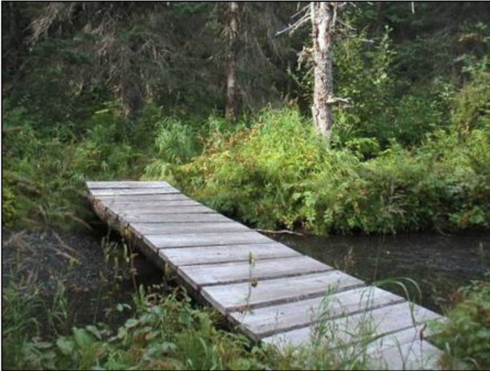
Structure has all the basic structural elements and is over actively flowing water.
