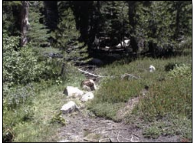
Figure D-5—Rocks and logs were installed on social trails and closed campsites to deter use and provide microhabitat for plantings.
