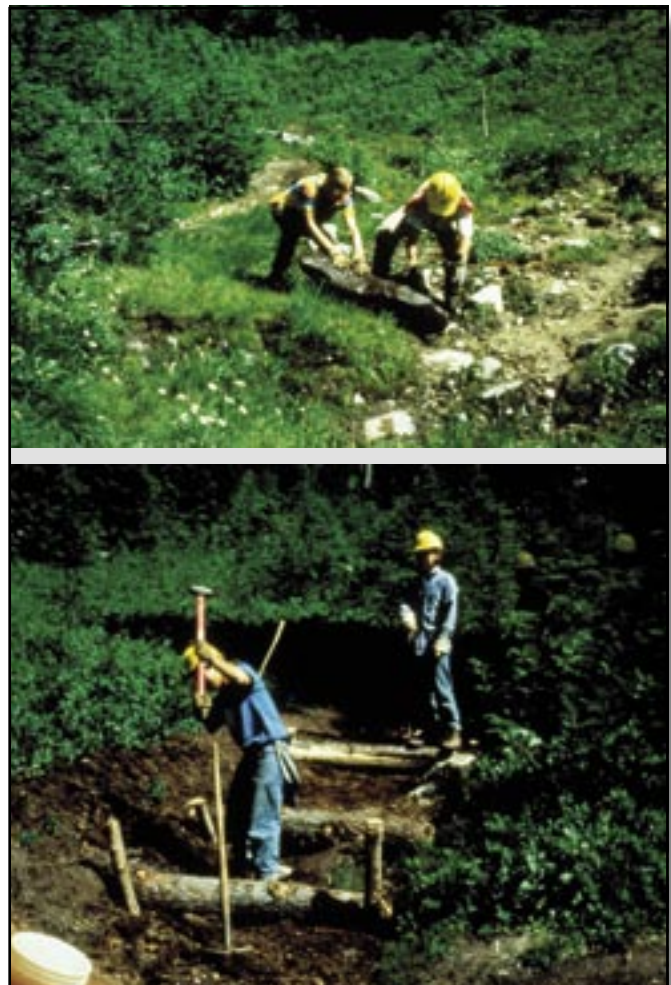
Figures D-3a and 3b—Teenagers on a Student Conservation Association high school work crew spent many hours installing and backfilling rock (top) and installing log checkdams (bottom) to stabilize erosion at Lake Valhalla.
