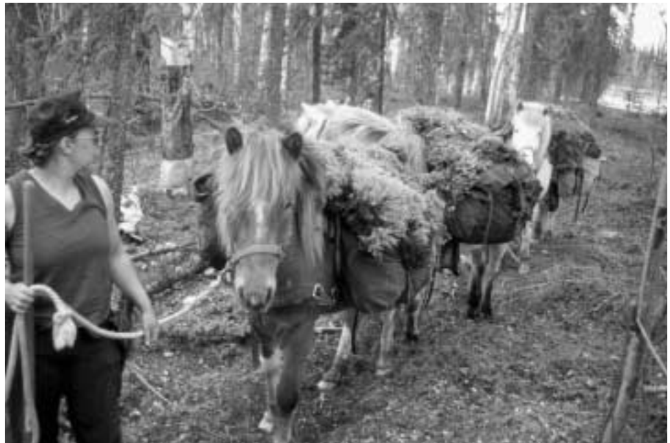
Figure 2—Moss makes good insulation on cabin roofs. Miki uses her Icelandic horses to pack moss to an old trapping cabin whose roof is being repaired. Photo courtesy of Miki and Julie Collins.
